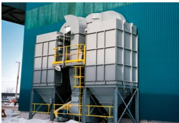
Two TubeJet collectors remove limestone dust from a utility scrubber dumping station. Each collector handles 11,000 ACFM.
