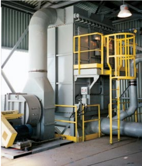
Limestone crusher and slurry mixer at a major coal-burning utility are ventilated by this TubeJet collector handling 10,000 ACFM .
